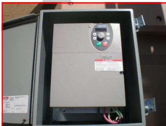
Electronics Enclosure housing the variable frequency drive system
